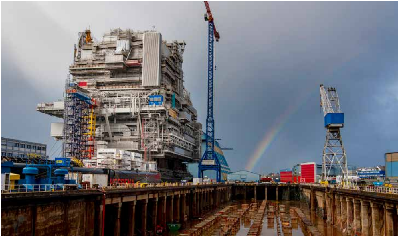
The P2 platform at Aibel's yard in Haugesund.
