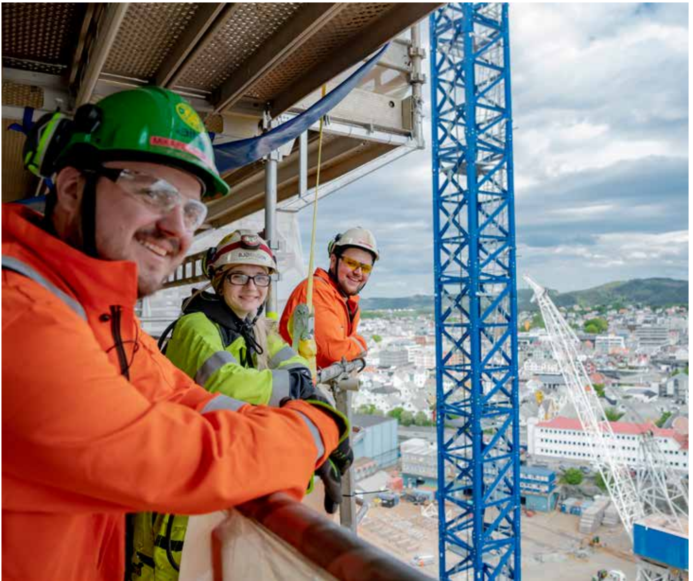
Mikael Kvinnesland, Ingrid Brekke Bjørnsen and Mats Søvik all work as welders on the P2 platform.
